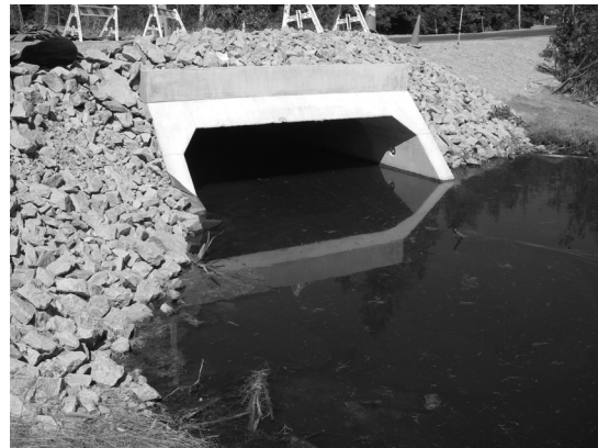
Figure 11. The upstream side of the same crossing after replacement. Photo Credit: Merry Gallagher.
