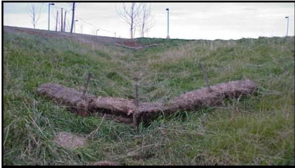
Vegetated swale with hay bale check dam to reduce velocities under construction.
