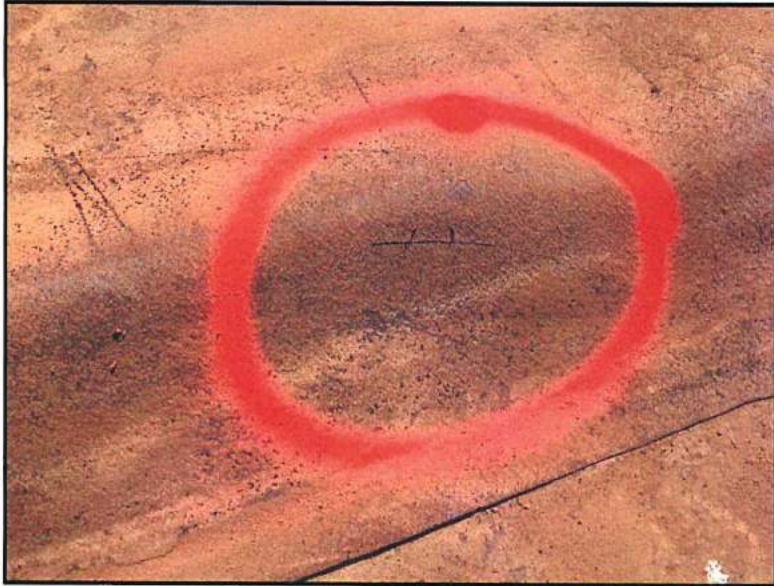
Scratch (Damage Location 6)
