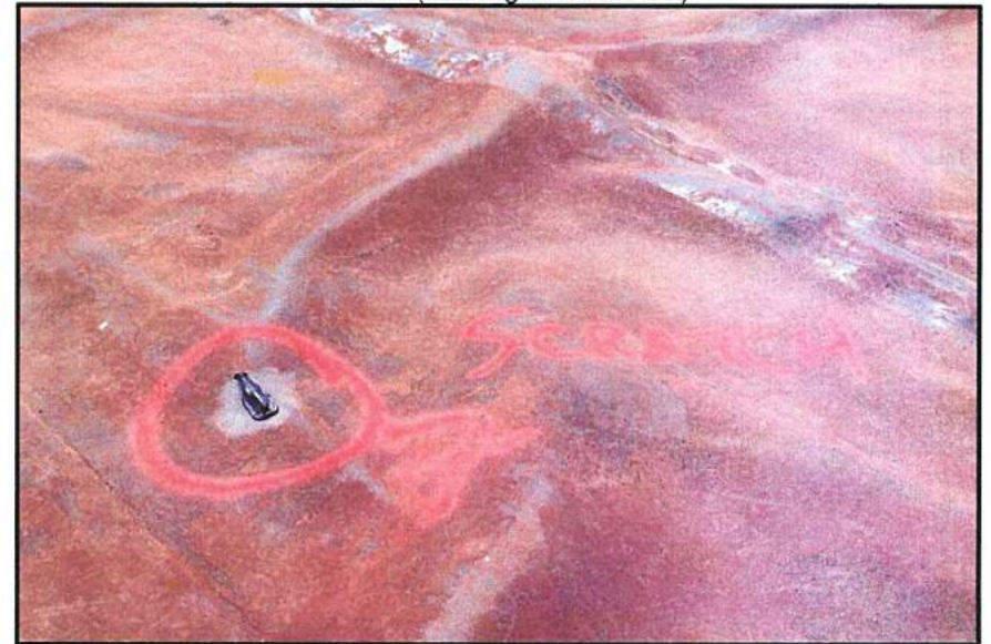
Repair (Damage Location 7)
