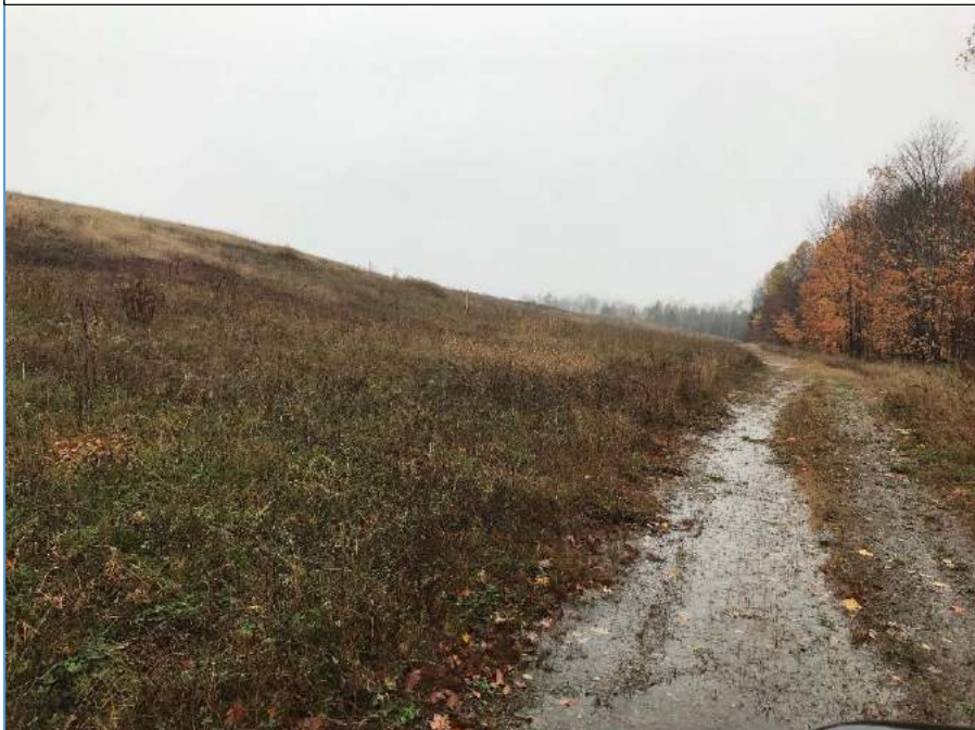
DOLBY II COVER SYSTEM – EAST SIDE
