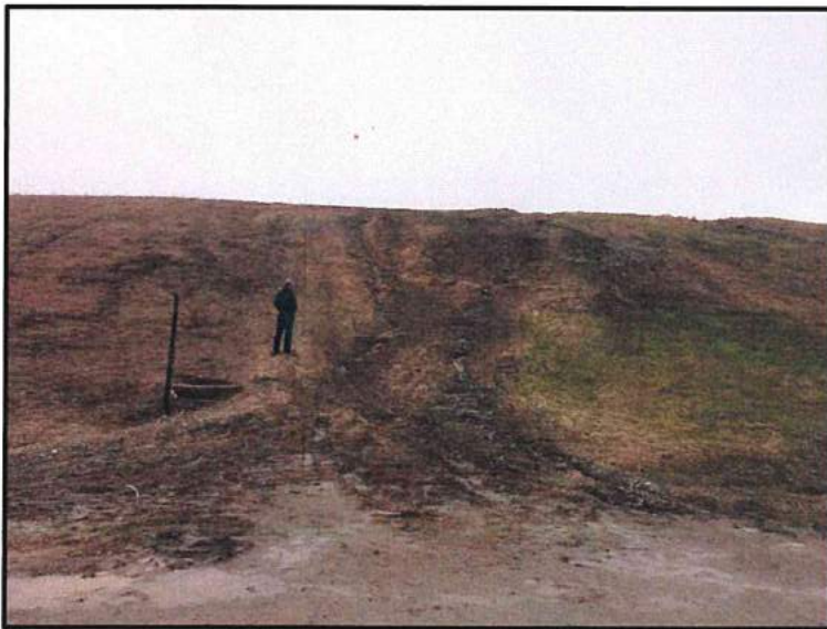
Slope erosion on south end of west slope.
