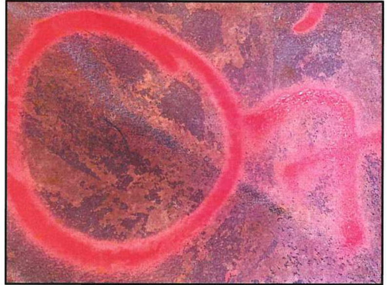
Scratch (Damage Location 7)
