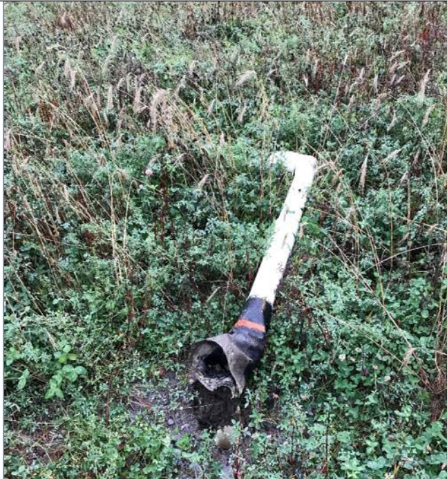
DOLBY III BROKEN GAS VENT ON TOP OF PHASE I COVER UPGRADE AREA
