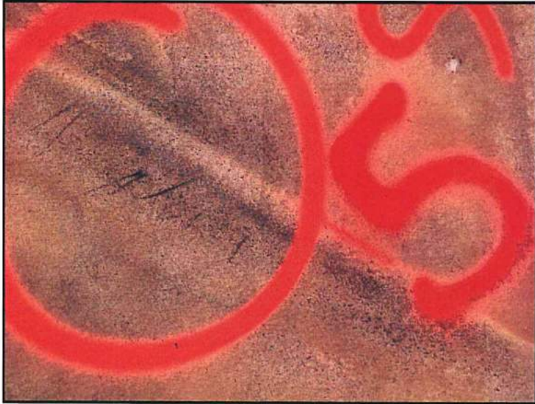
Scratch (Damage Location 5)
