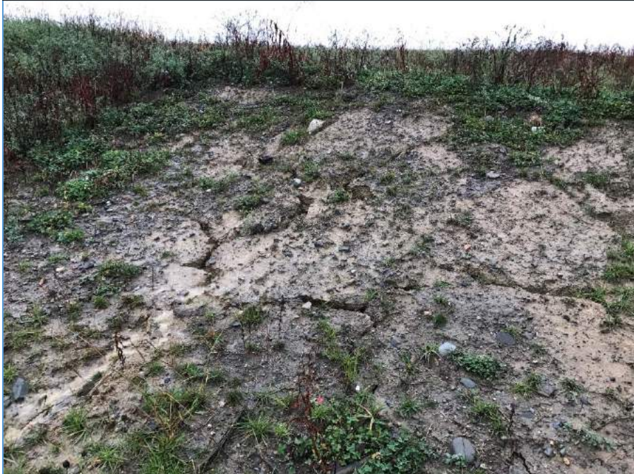
DOLBY III AREA OF SOIL EROSION AT TOP OF SOUTHERN- MOST DOWNSPOUT ON PHASE I COVER UPGRADE AREA
