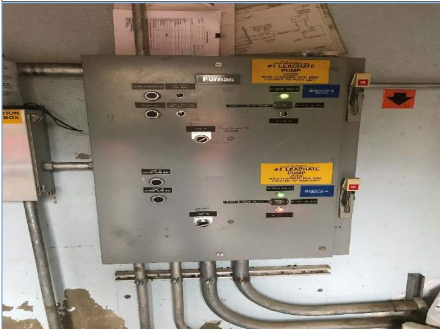
LEACHATE PUMP STATION CONTROL PANEL
