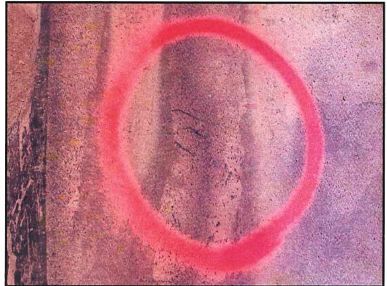
Scratch (Damage Location 6)
