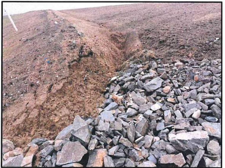
Erosion at Phase I cover upgrade area. Slope terrace/downspout transition.
