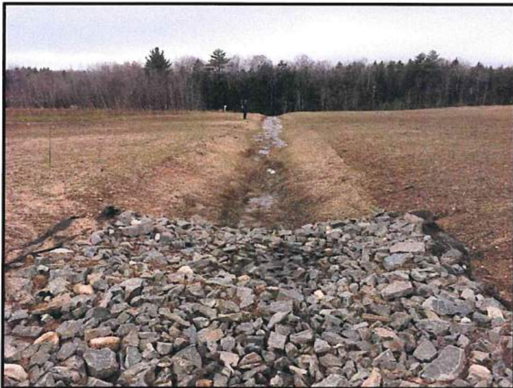
Erosion in Phase I cover upgrade grass downspout.
