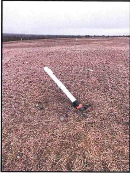
Broken gas vent on Phase I cover upgrade area.
