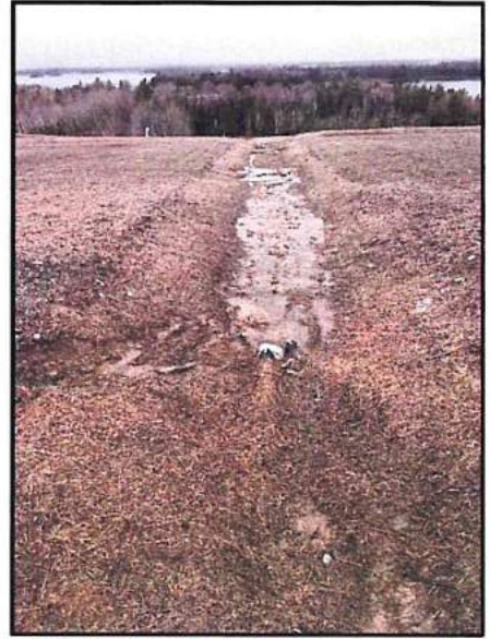
Erosion at Phase I cover upgrade grass downspout.
