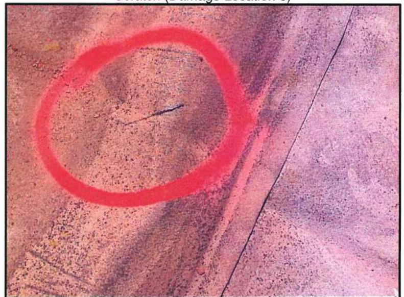
Scratch (Damage Location 6)
