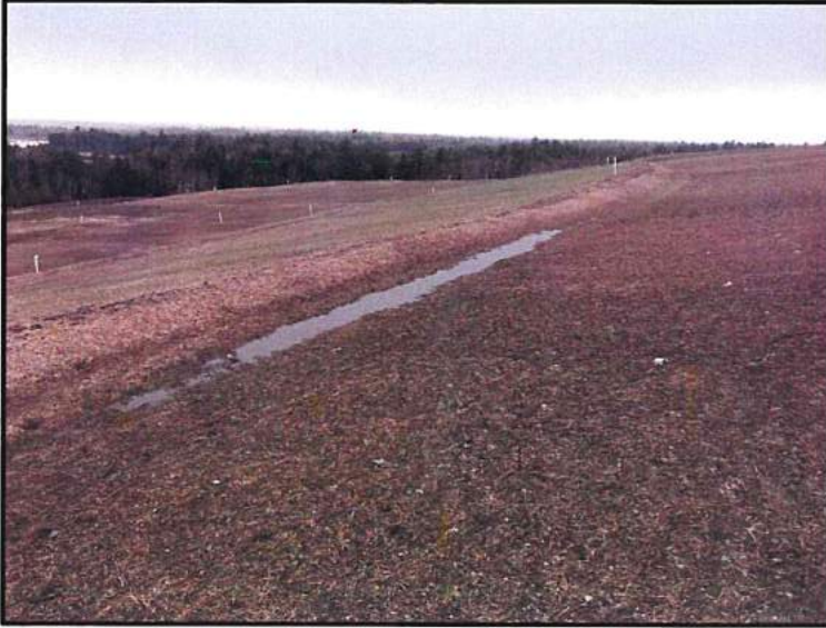
Ponded water observed in upper terrace Phase I cover upgrade area.
