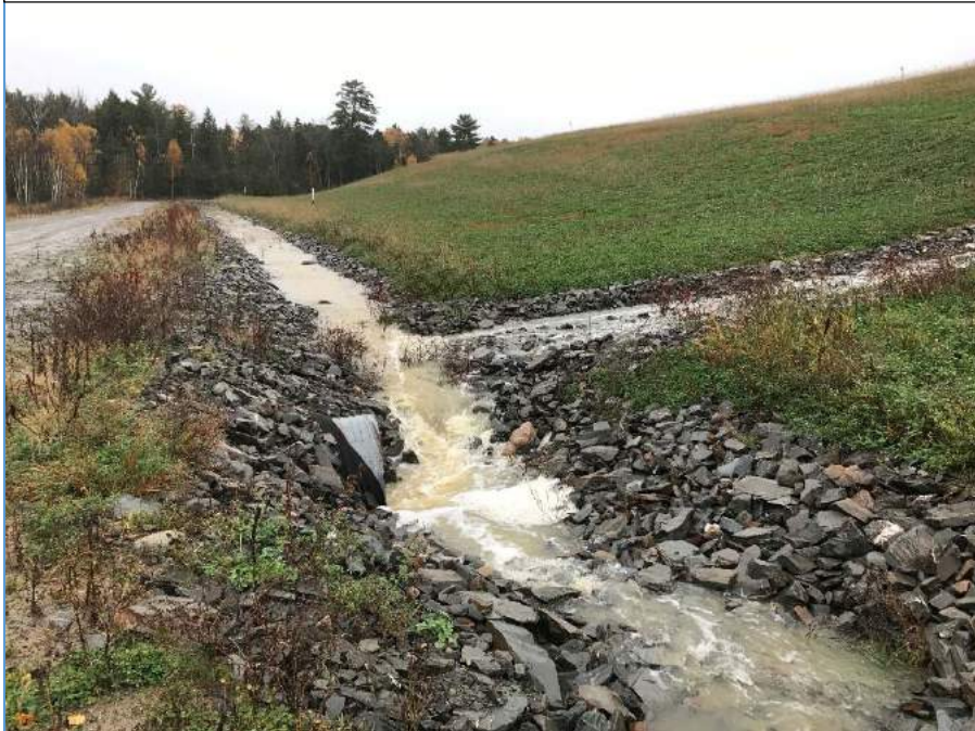
DOLBY III TOE DITCH AT WESTSIDE OF PHASE I COVER UPGRADE AREA
