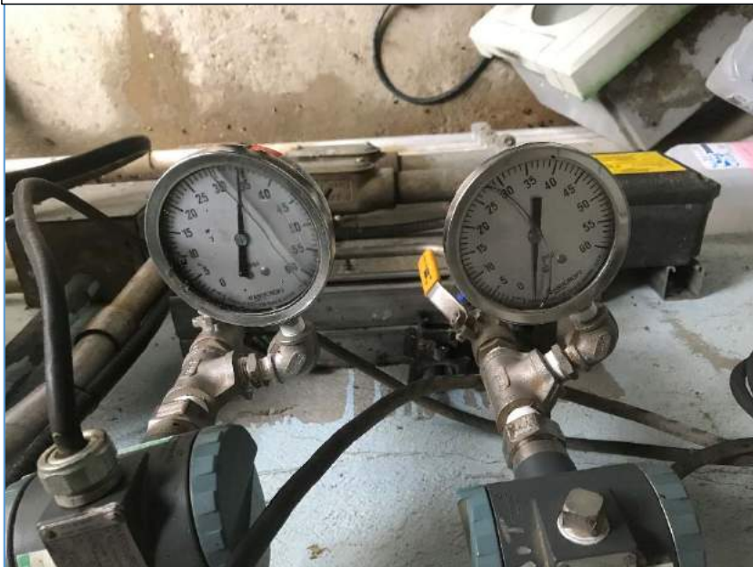
LEACHATE PUMP PRESSURE GAUGES
