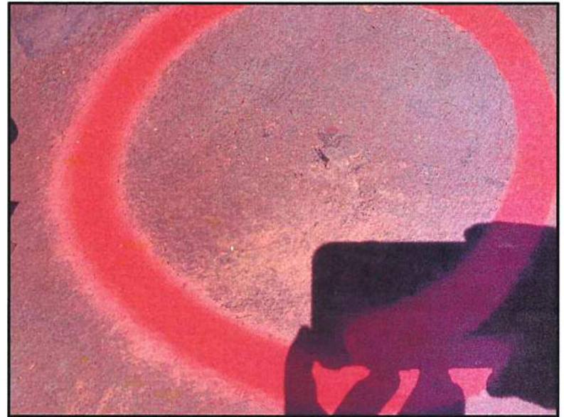
Hole (Damage Location 2)
