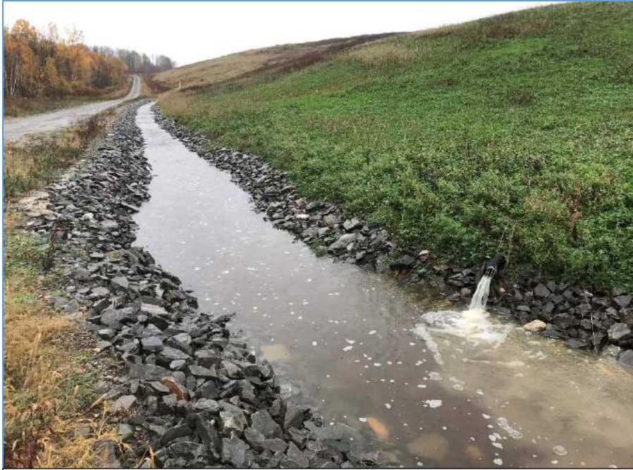
DOLBY III TOE DITCH ON NORTH SIDE OF PHASE I COVER UPGRADE AREA
