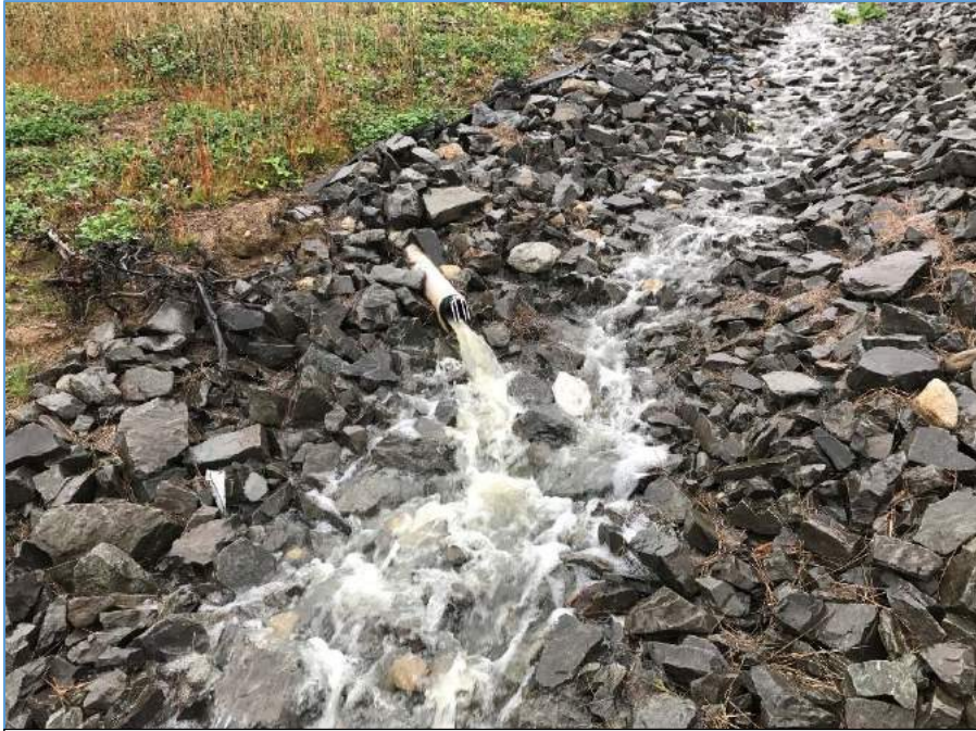
DOLBY III RIPRAP DOWNSPOUT AND COVER DRAIN ON PHASE I COVER UPGRADE AREA
