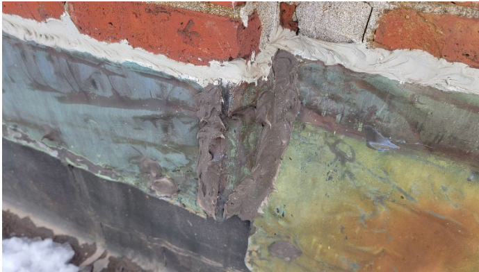
Photo 3 (12/21/2022): Black roof sealant on Roof Area B testing positive for asbestos (sample set 008). Gray caulk above was negative for asbestos (sample set 007).
