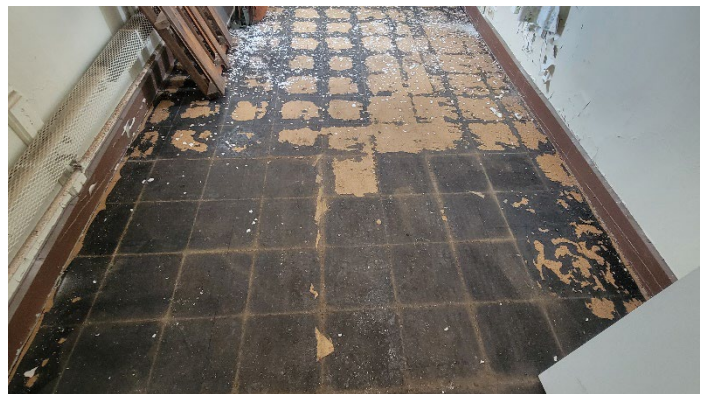
Photo 6 (March 9, 2023): ACM mastic (sample set EW-05) located on the interior of the north branch of the elevated walkways.
