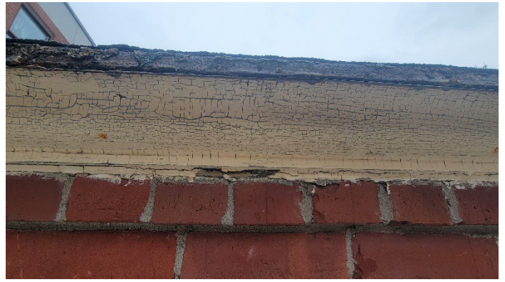
Photo 2 (March 9, 2023): ACM caulking (sample set EW-02) present between the wood trim and brick wall along the perimeter of Roof Area D2.
