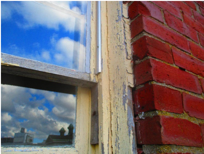
Photo 5 (March 9, 2023): ACM window caulk (sample set SKY-04) located between window casings and brick wall on the elevated walkways.
