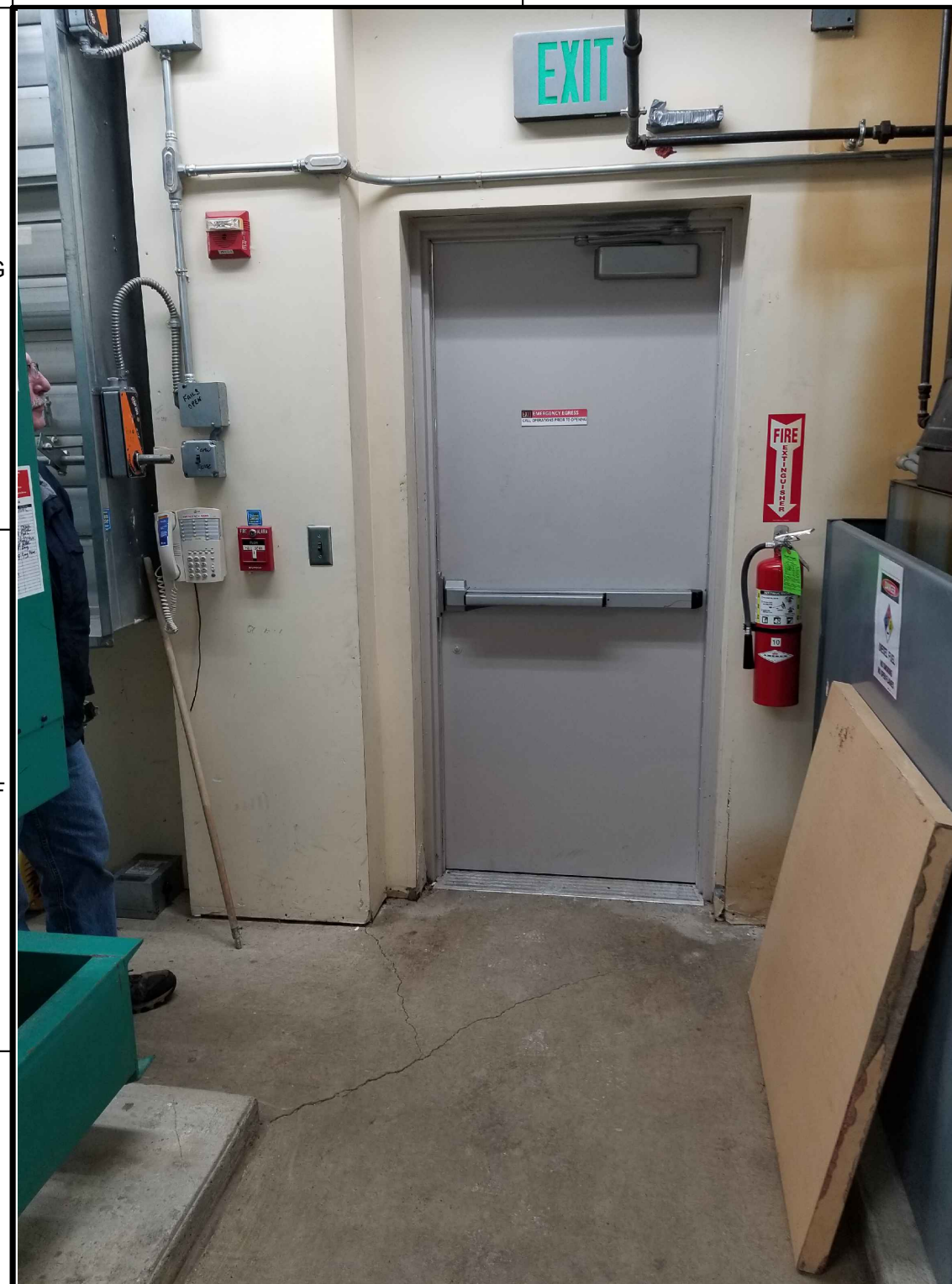
E1 PHOTO #1 - ENTRY FOR EQUIPMENT DO NOT SCALE
