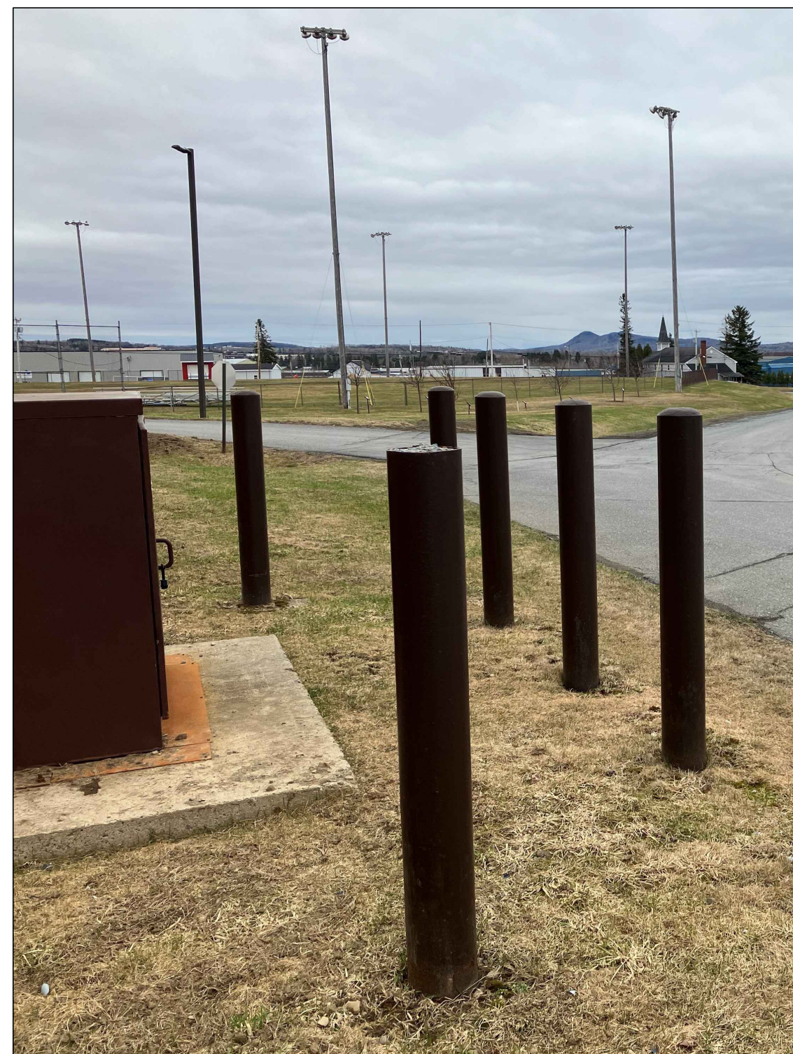
D3 EXISTING PAD MOUNT TRANSFORMER
