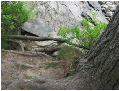
BLUFF EROSION AND LEDGE ARMOR
