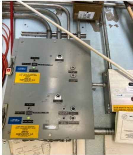
Leachate Pumpstation Control Panel
