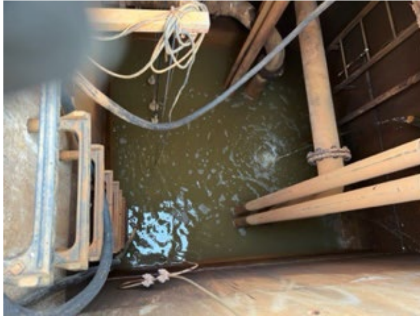
Pumpstation Wet Well
