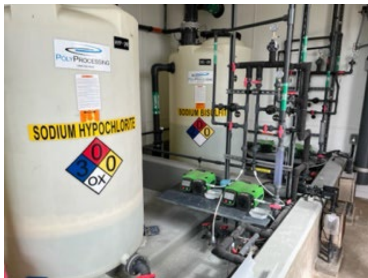
NaHSO 3 and NaOCl Tanks
