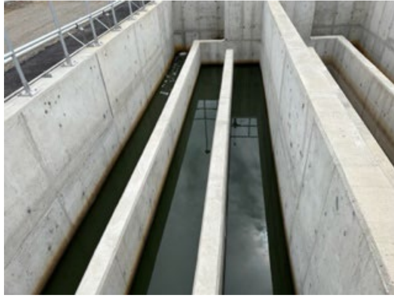
Cl2 Contact Tank
