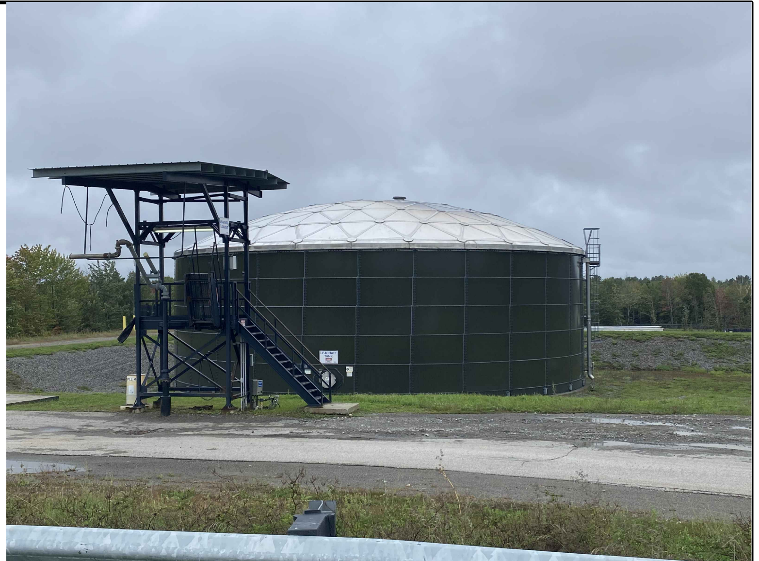
LEACHATE TRUCKED 7 MILES TO TREATMENT PLANT LEACHATE LOADING RACK AND TANK
