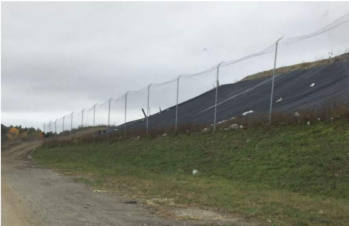
17. at the southern toe of the landfill looking southwesterly along the south face of Cell 10
