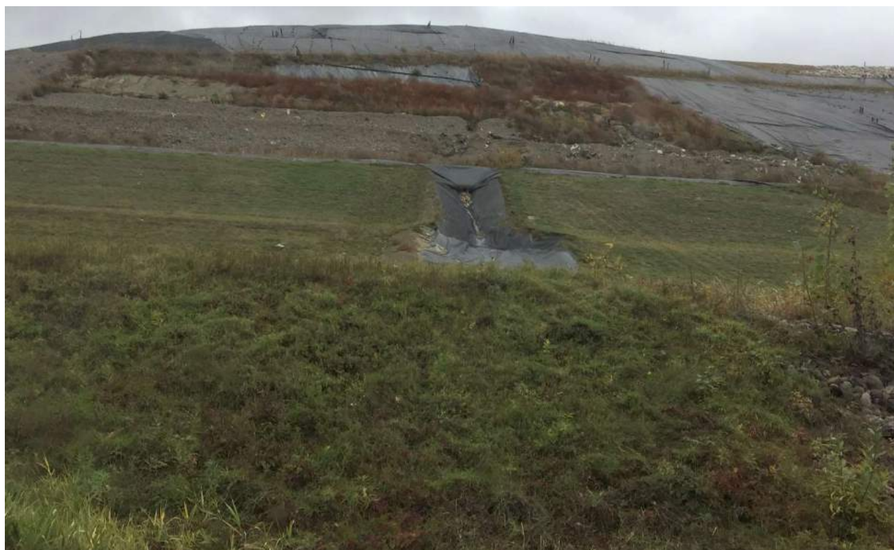
6. at landfill toe looking east up the western slope of Cells 1 & 2 (the location of the previous excavation area)
