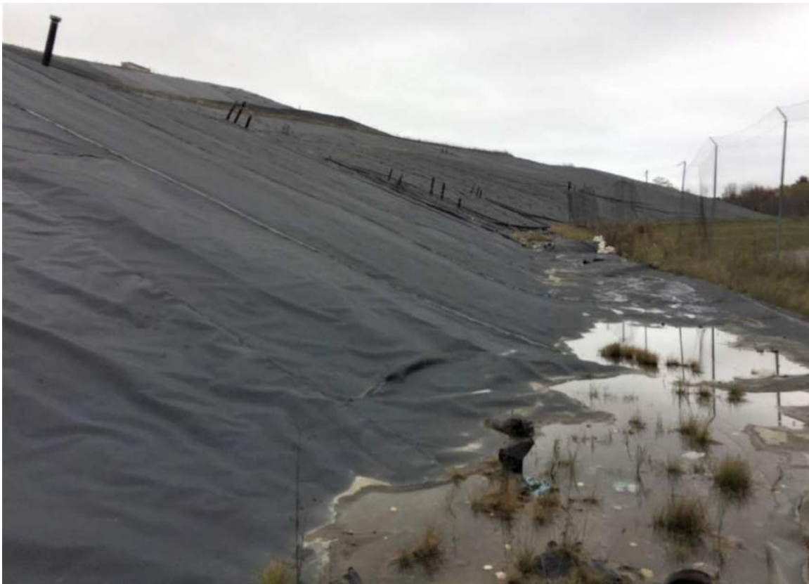
13. looking southeasterly along south face of Cell 4/5 towards southwest face of Cell 5/6
