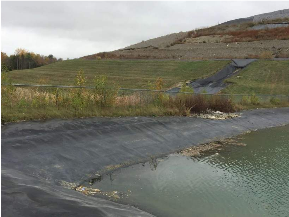
7. at western detention pond looking north towards bottom slope of Cell 1 & 2 (and northern portion of the excavation area)
