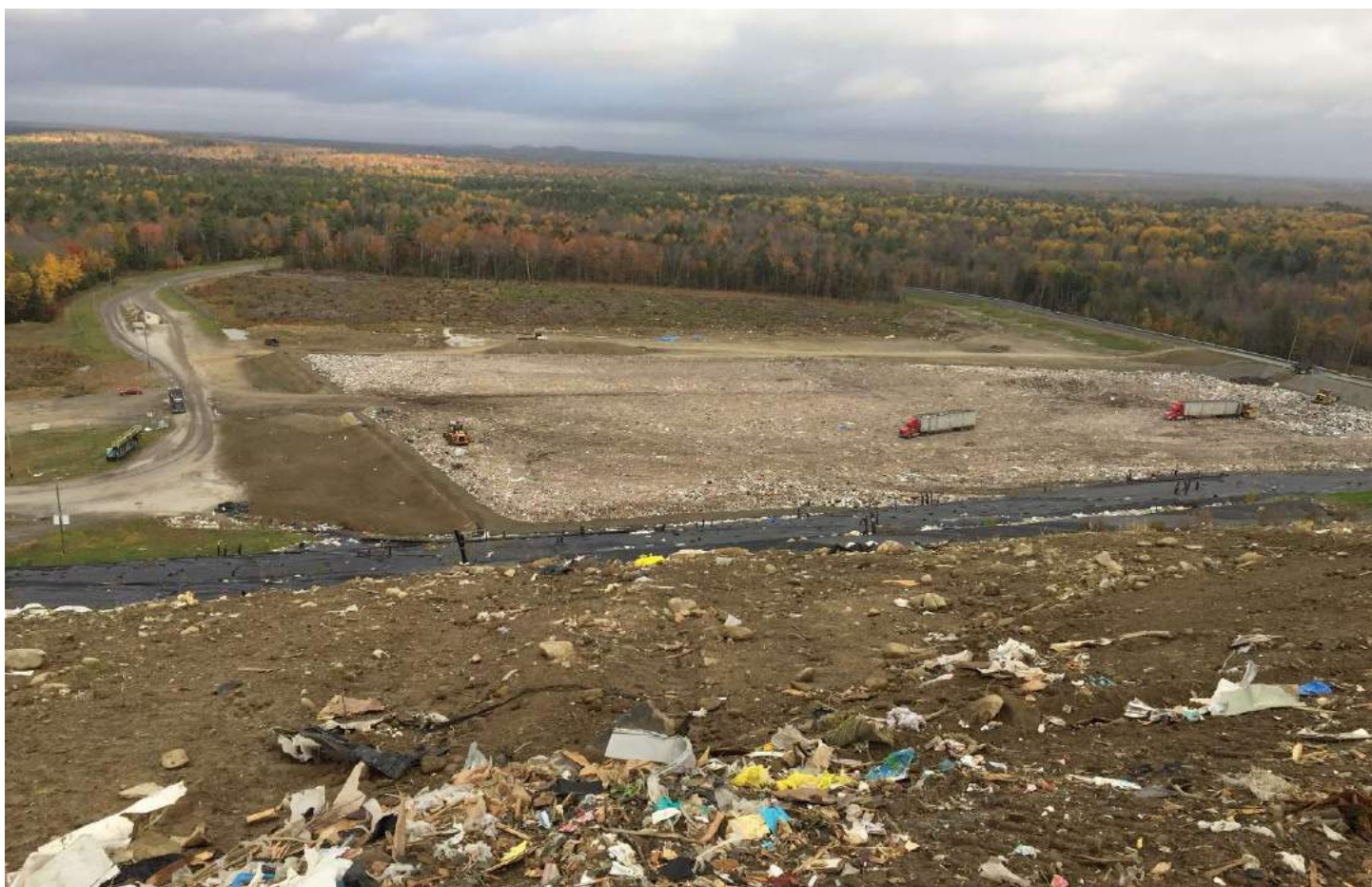
26. top of landfill looking northerly down north slope towards the soft material placement into Cell 12
