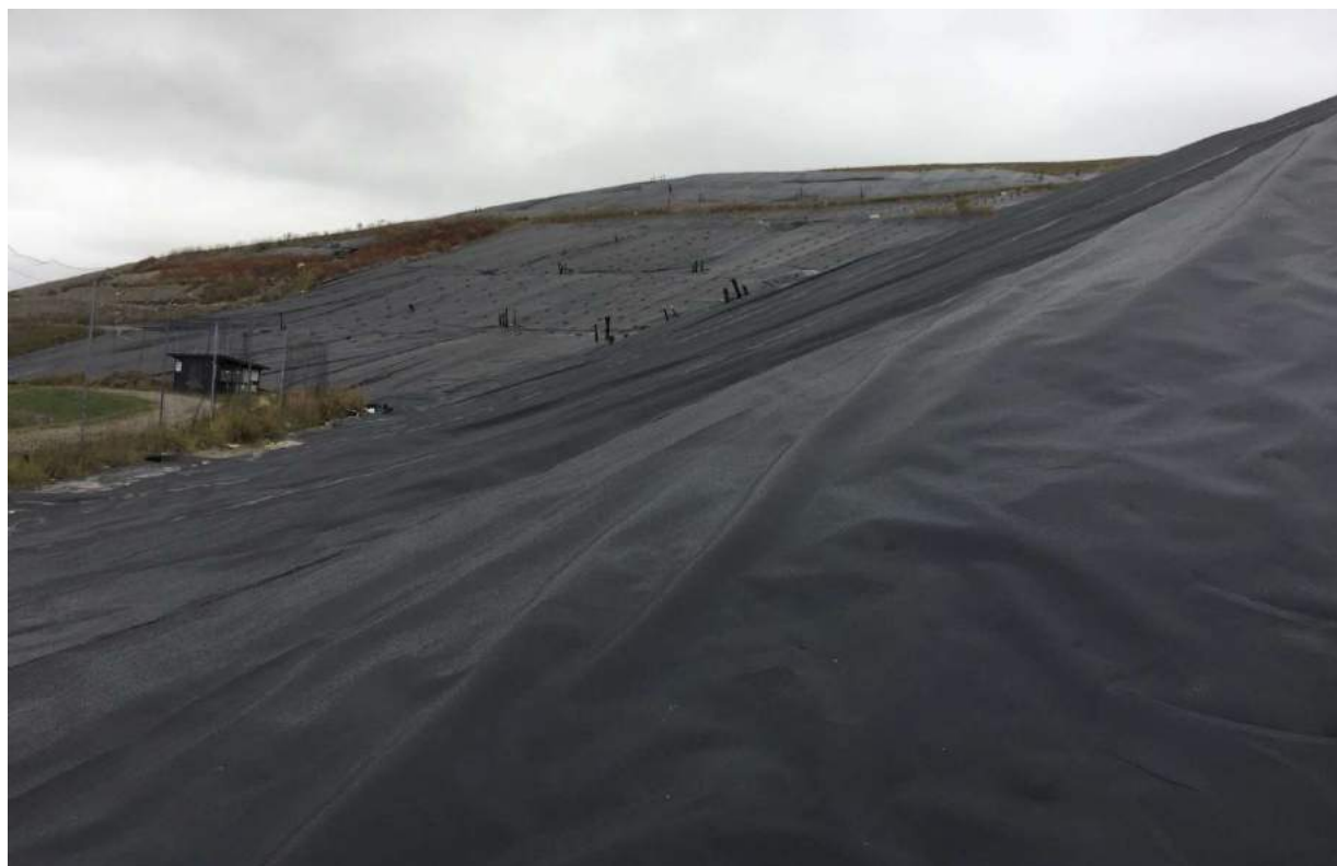
12. looking northerly along west slope of Cells 4/5 to southeast slope of Cells 4, and 1/2
