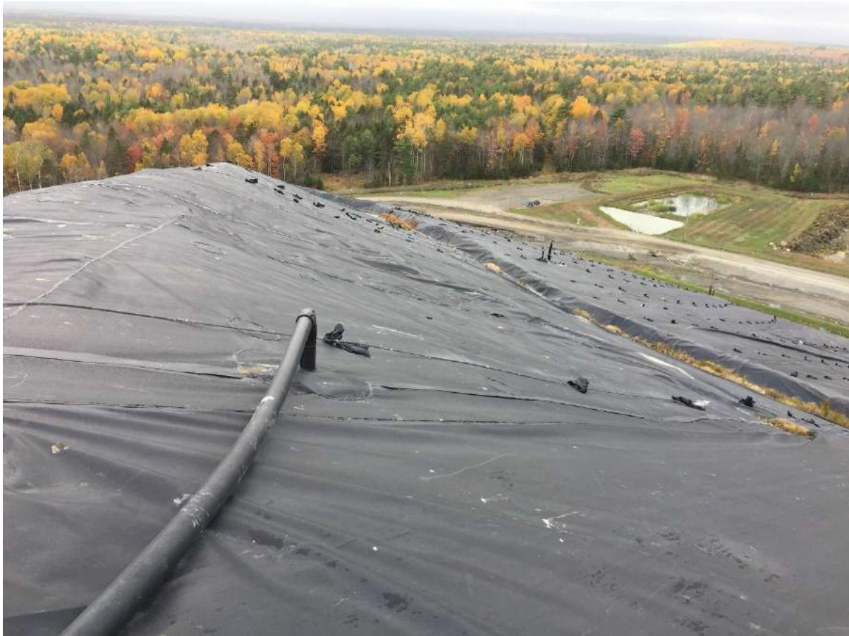
3. looking northwesterly along western portion of the northern slope in the transition between Cell 3 & Cell 1 & 2
