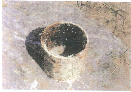
Photo 1. Infiltration pipe in test pits TP-2 and TP-3 not blocked.
