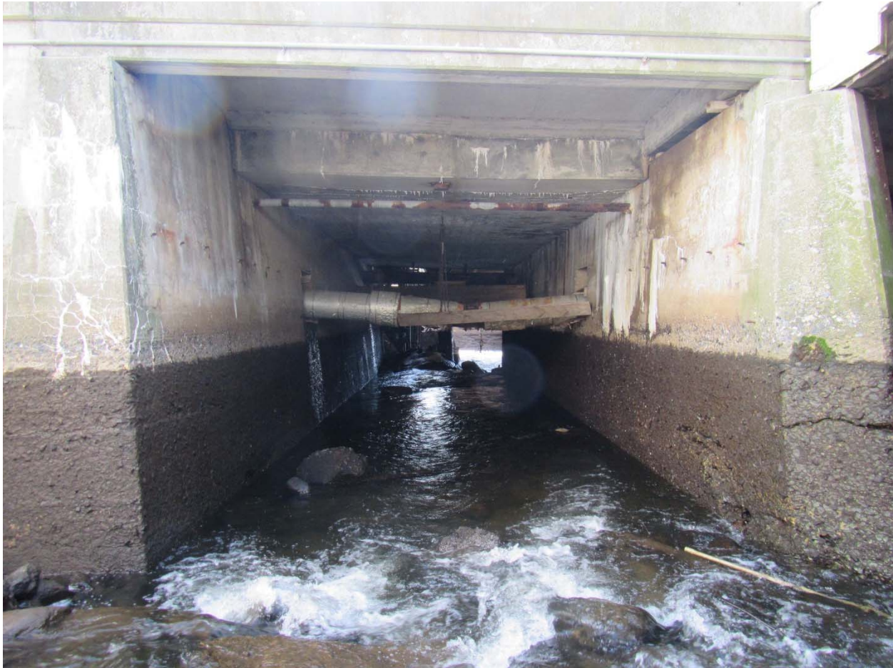
Figure 25. View downstream through north span of Main Street bridge in drawn down condition, May 8, 2018. Stain lines indicate normal pool elevation.
