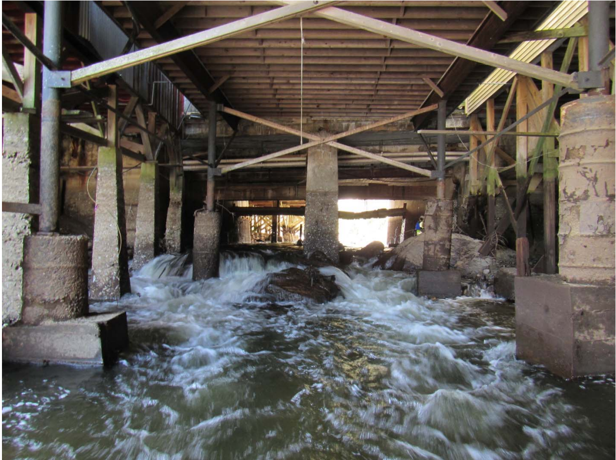
Figure 26. View upstream at Main Street bridge in drawn down condition, May 8, 2018. Hydraulic drop at downstream bridge opening in center of photo. Stain lines apparent on posts indicate normal pool elevation.
