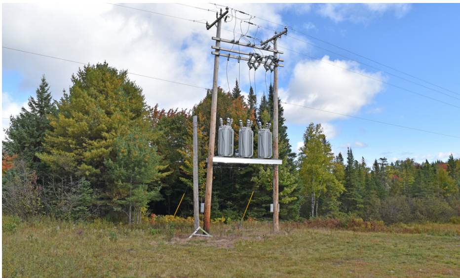
Photograph 13: Transmission line structure at the intersection of the Jackman Tie Line and Route 201 in West Forks Plt.
