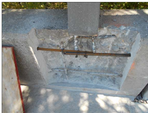
Figure 6 - Typically a concrete base repair would be focused beneath or partially beneath a rail post.
