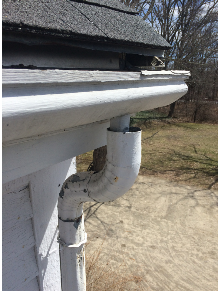
This wooden gutter at the Parson Smith House has an undersized outlet made of metal. It was found that most of the historic wooden gutters had undersized outlets. Photograph taken by Shawn Beckwith, April 18, 2018.
