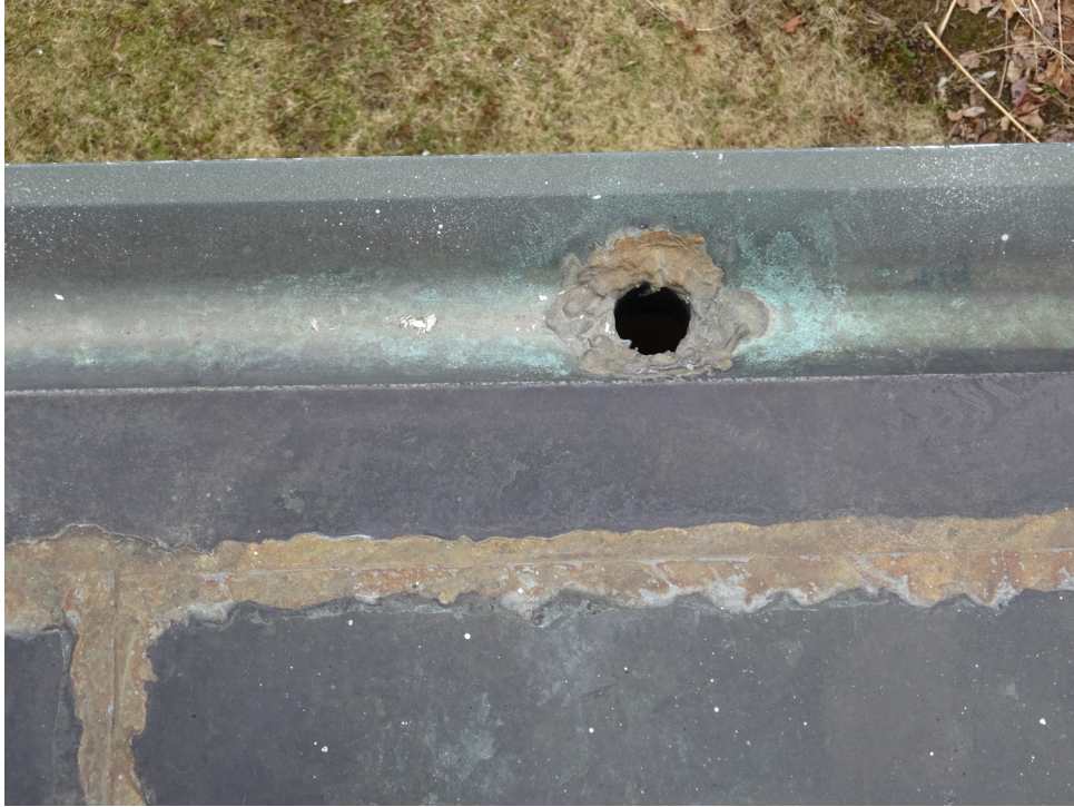
Above: A build-up of solder around this outlet is hampering water flow. Soldered joints should be smooth so the water can flow into the outlet. Photograph taken by Margaret Gaertner, April 20, 2018.
