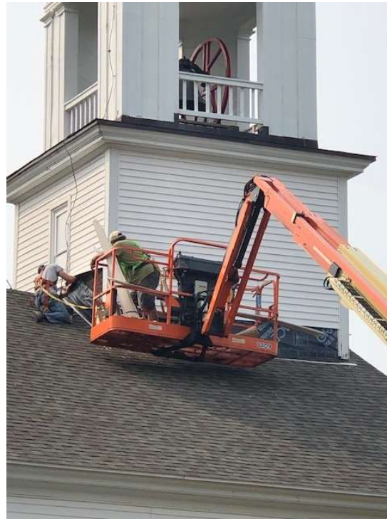
Replacing tower box siding at the Bell Hill Meeting House, Otisfield in 2021. Photograph by Ken Bartow.
